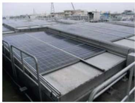
Solar powered system
