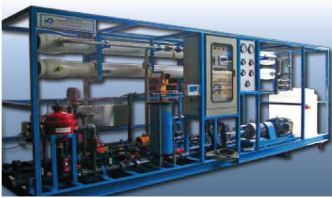
100,000 litres/day production capacity Seawater RO powered completely by solar power in Abu Dhabi, UAE
