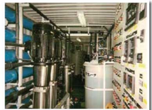
Containerized RO system
