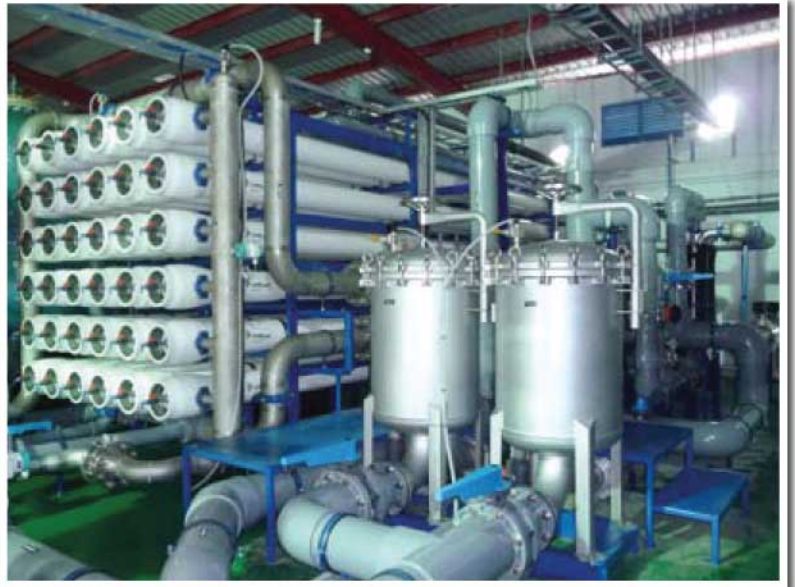
3,000,000 litres/day production capacity Seawater RO in Male' Republic of Maldives
