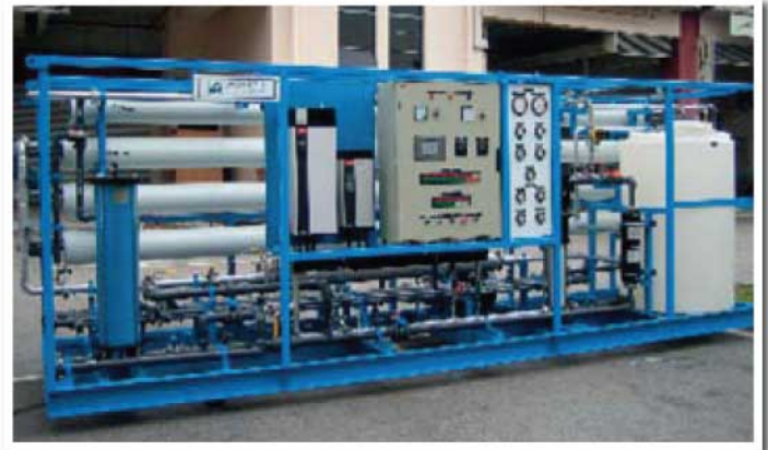
200,000 litres/day production capacity Seawater RO with PX Energy Recovery Device in Zanzibar, Tanzania
