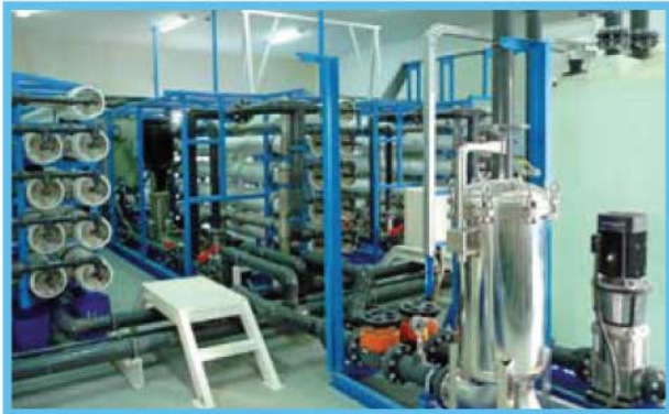
3,000,000 litres/day production capacity MBR-RO in Dubai, UAE
