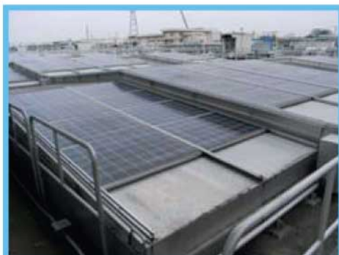
Solar powered system
