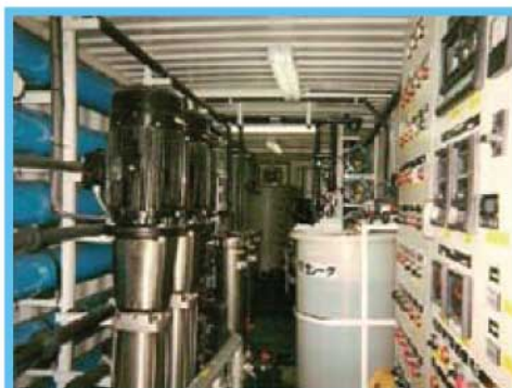
Containerized RO system
